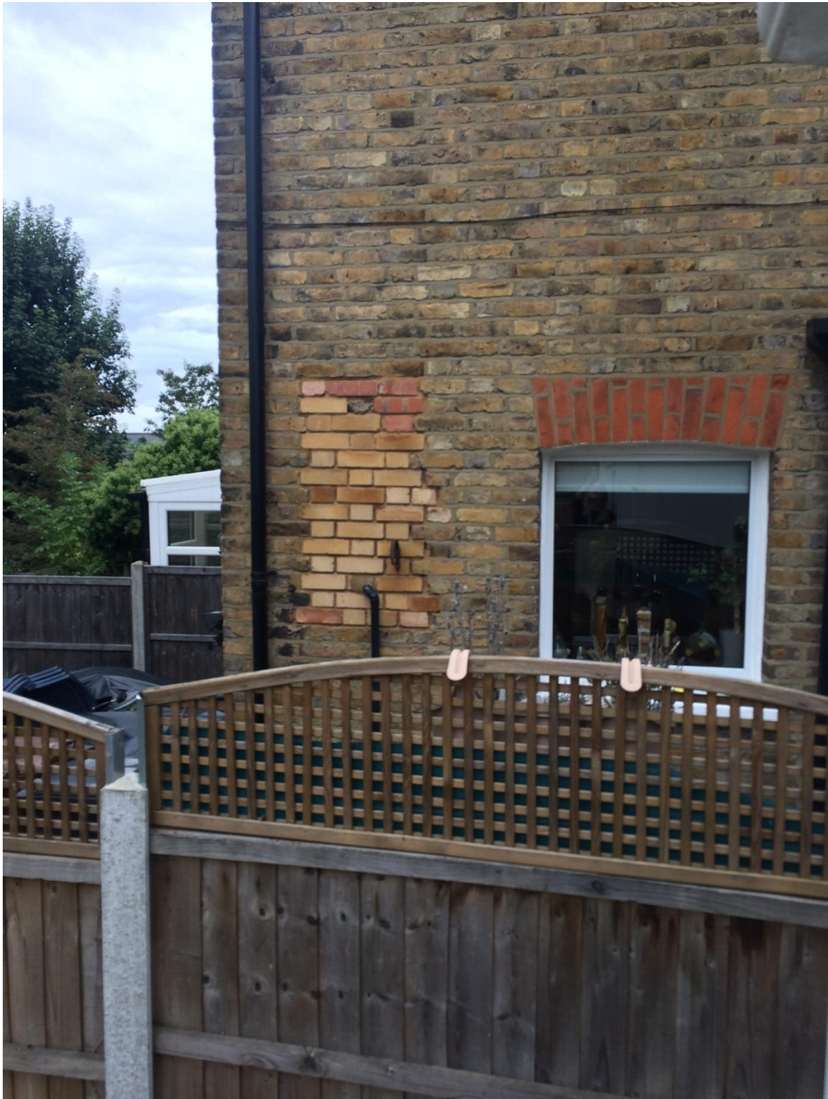
Figure 4 Flank elevation of the outrigger on No. 40 Roxeth Hill, taken from the rear steps of the existing rear extension
